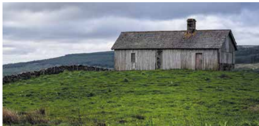
Figure 3 The Eilean nan Caorach Geala Research Centre. The building itself is in need of some substantial renovation
