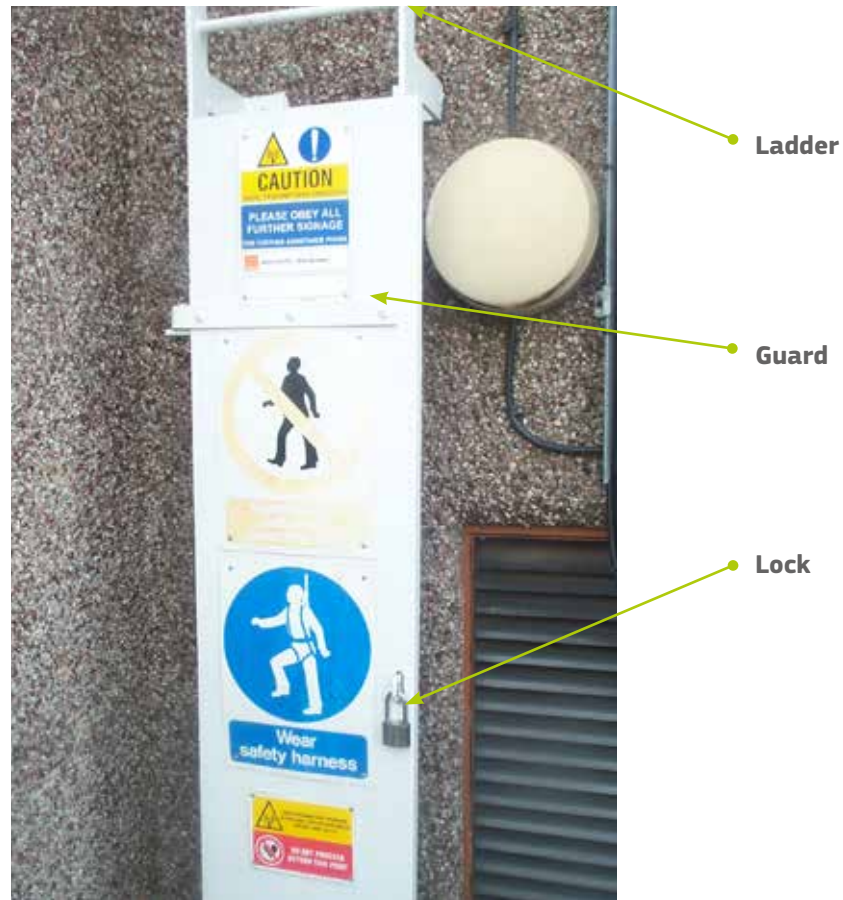
Figure 9.2 — Use of ladder guard to restrict access to strong fields on a rooftop
