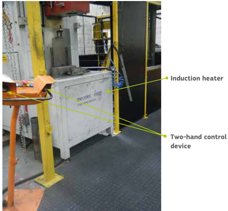
Figure 9.4 — Two-hand control device used to ensure worker separation from induction heater
