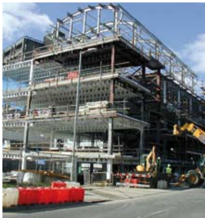
Building work well underway on the new research centre earlier this year.
